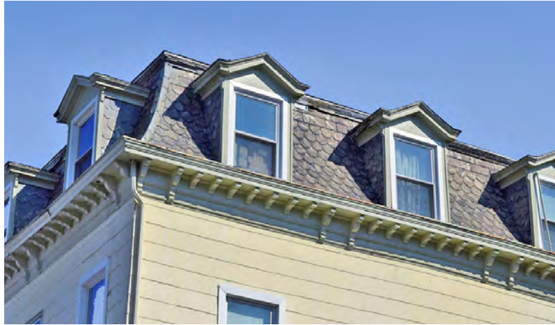
The fishscale-pattern slate on this Mansard roof is largely intact and important to the building's historic character.
