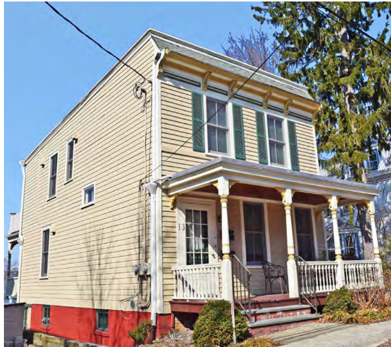
A low-slope roof like that on this marvelous residence can be re-roofed with any contemporary material but visible flashings and gutters should be carefully selected.
