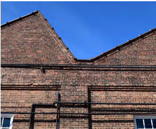
Classic sawtooth brick structure provides a profile and texture to be maintained.
