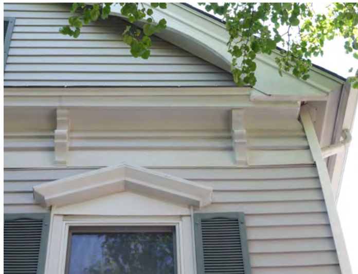
Brackets, window hoods and cornices should be repaired with epoxy consolidant or other techniques if possible. Fiberglass or similar substitute materials may be acceptable if they take paint or stain and are indistinguishable from the original from normal viewing locations.
